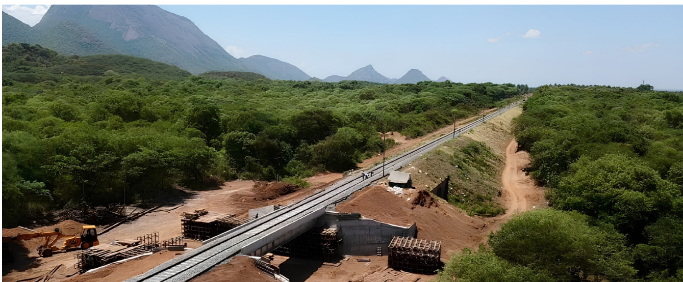
Figure 6. Railway underpass constructed to facilitate safe elephant movement along the Ettimadai–Walayar railway section in Tamil Nadu (Photo credit: Tamil Nadu Forest Department).
